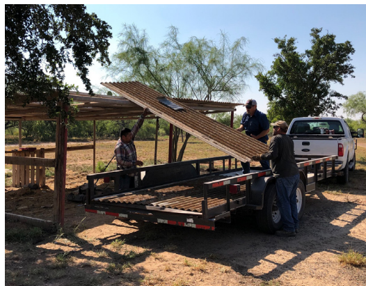
The Field Operations team, Rafael Guerra, Jason Haynes, and Sergio Vasquez work together to dismantle a lean-to shed.
